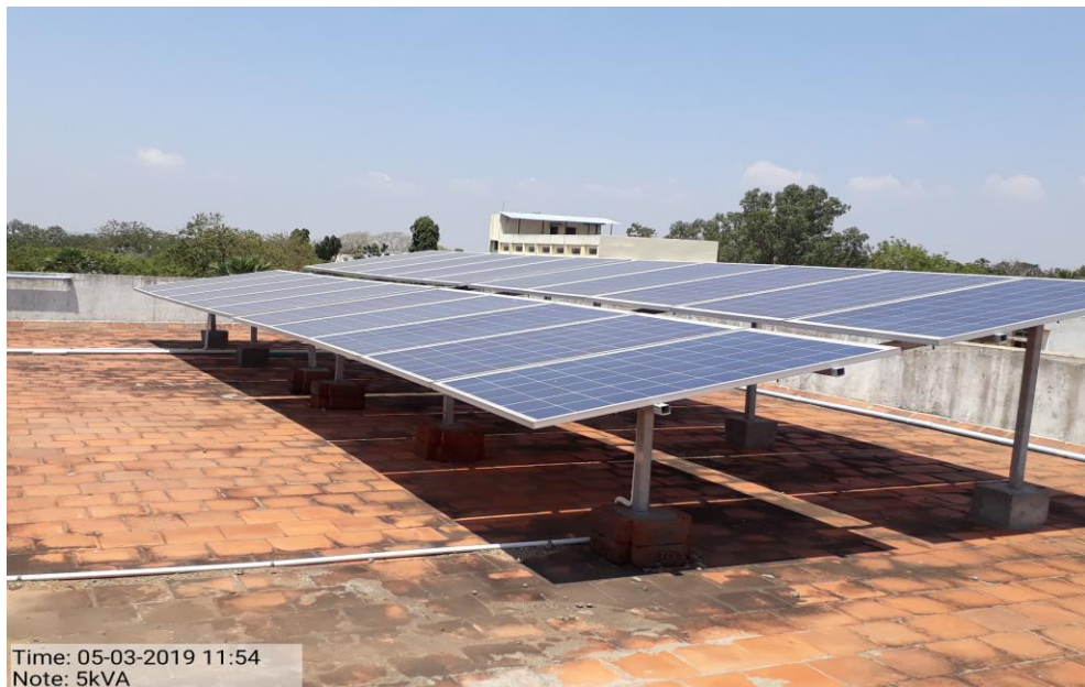
Photo-3 Solar Plant
